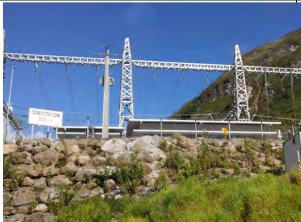
Photo 23: Substation on site
