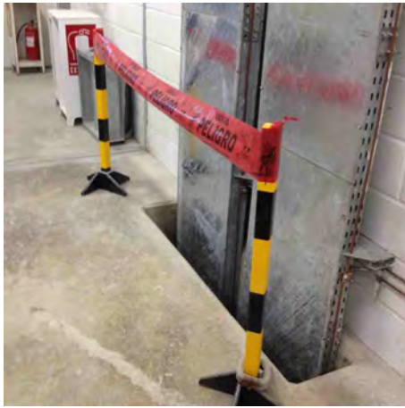
Photo 73: Example of temporary hazard barriers at the powerhouse
