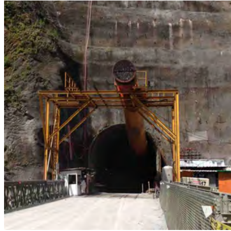
Photo 116: Air extraction system seen at one of the adits to the tunnelling
