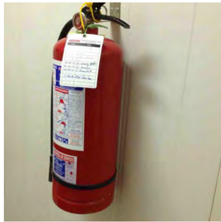
Photo 76: Fire-fighting equipment seen in dormitory blocks
