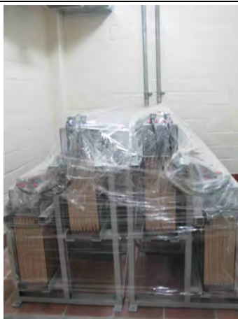
Photo 17: New batteries in powerhouse
