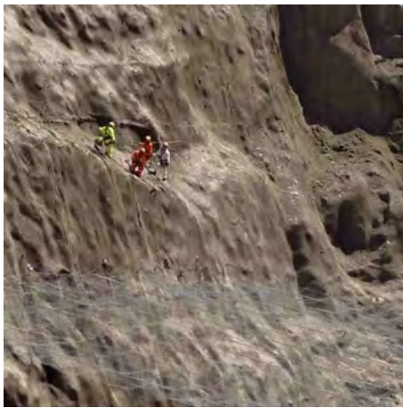
Photo 69: Employees working at height with hard hats and netting, at the small hydropower station
