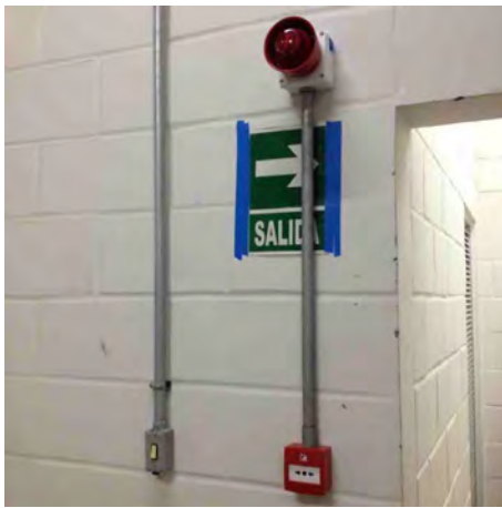
Photo 75: Fire alarm systems installed at the powerhouse, and temporary signage
