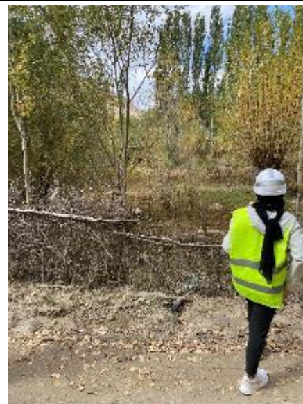
Photo 107: Existing road, requiring rebuilding due to impoundment
