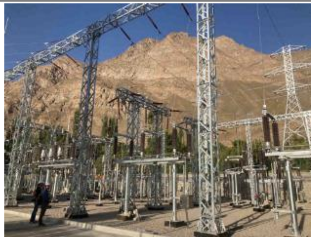
Photo 77: New 110kv substation at Khorog HPP
