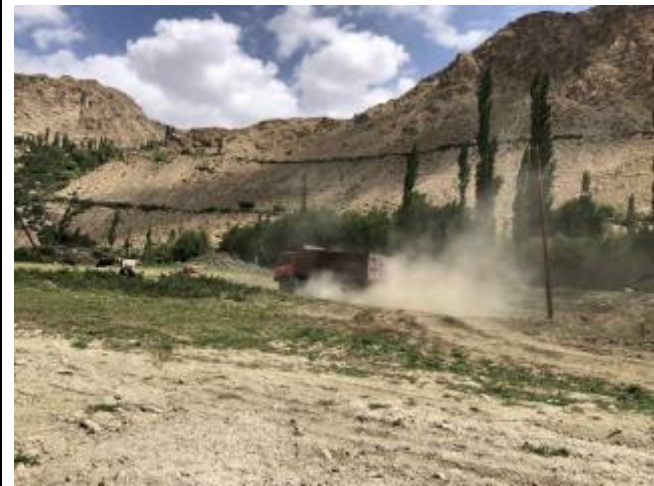
Photo 35: Construction traffic dust at intake
