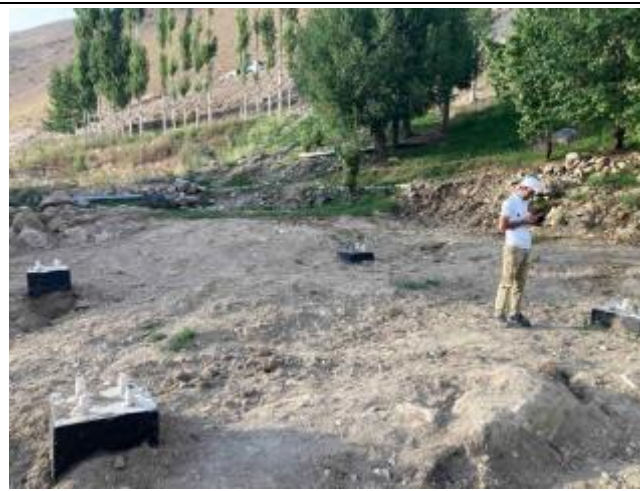
Photo 74: Transmission line tower foundations in Upper Chagev
