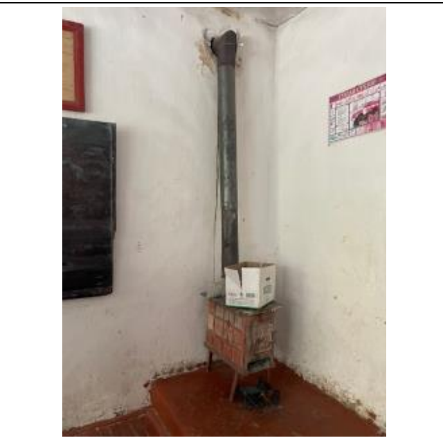
Photo 113: Traditional heating system used in existing school classroom
