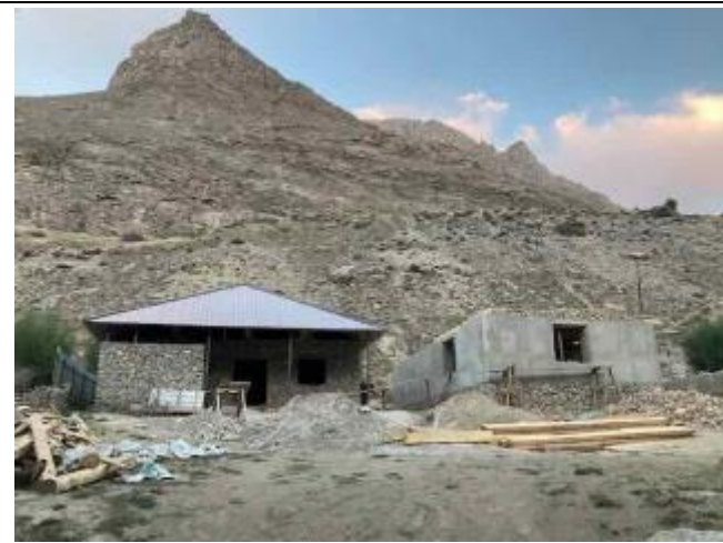
Photo 100: Replacement homes for homes destroyed in avalanche, funded by PEC and Ministry of Energy and Water Resources
