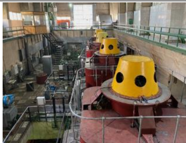
Photo 8: Pamir-1 HPP powerhouse
