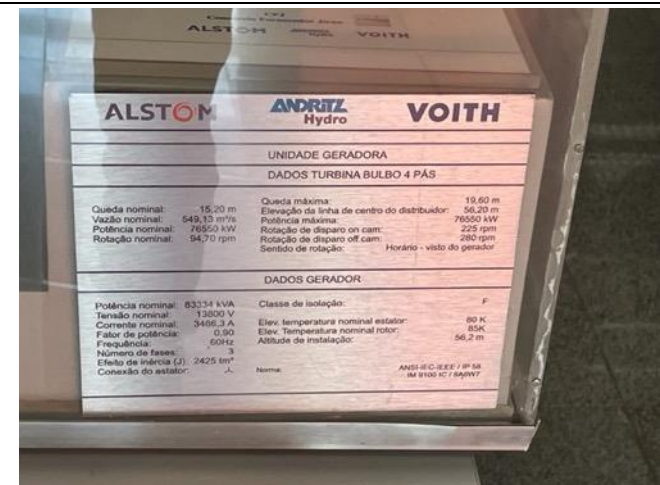
Photo 60: Turbine data right bank powerhouse
