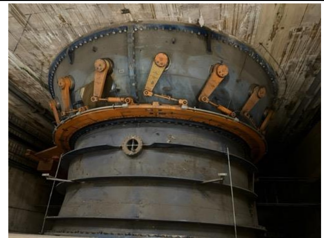
Photo 66: Bulb turbine distributor, view from above
