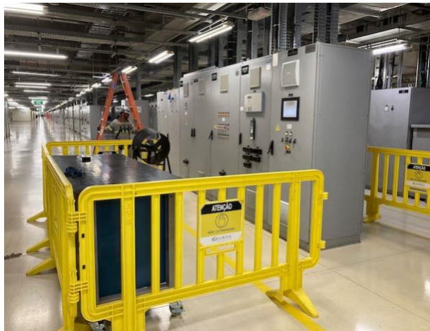
Photo 52: Safety barrier during electrical panel maintenance
