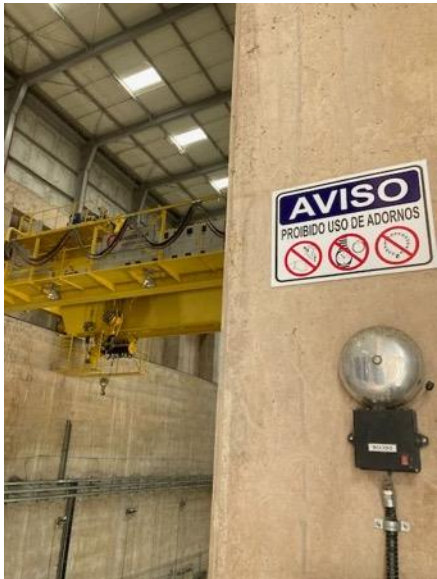
Photo 55: Alarm and warning signs in powerhouse
