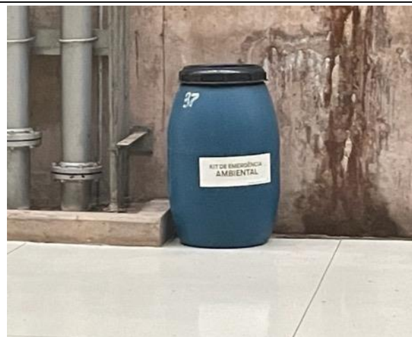
Photo 59: Spill kit in powerhouse
