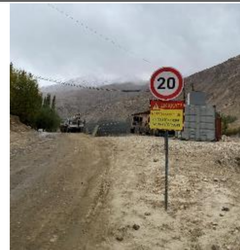
Photo 90: Speed restriction sign at the intake construction site
