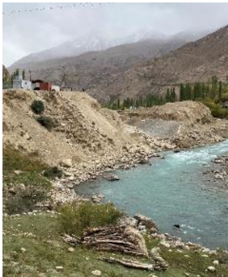
Photo 94: Unstable riverbank immediately downstream of the intake
