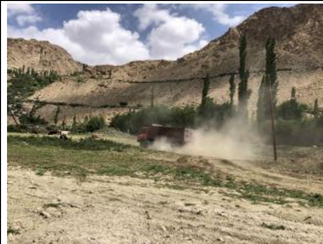
Photo 35: Construction traffic dust at intake
