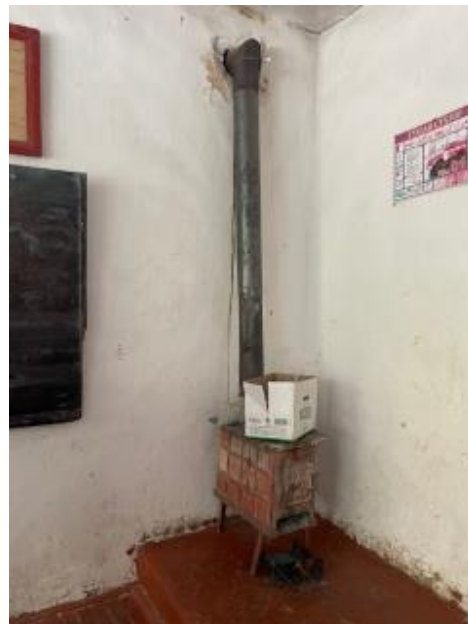
Photo 113: Traditional heating system used in existing school classroom
