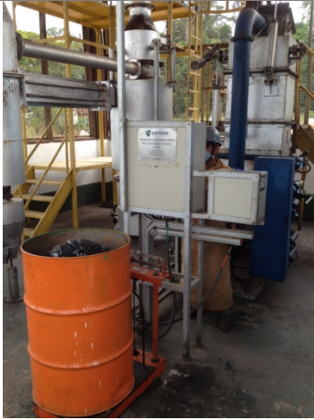
Photo 95: Incinerator at the waste processing centre.
