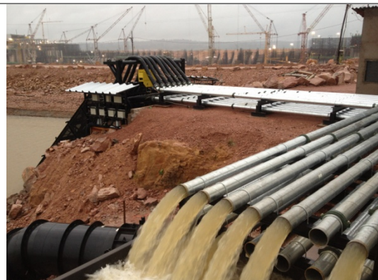
Photo 72: Fish passage pumps.
