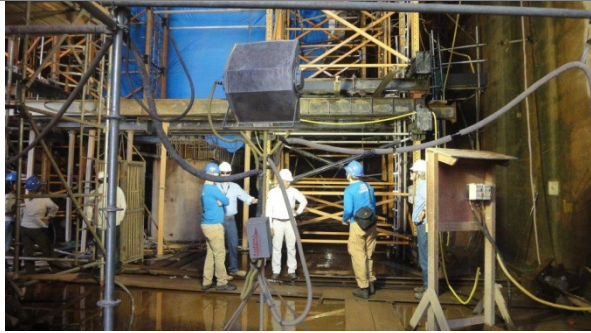
Photo 49: Inside Right Bank Power House - safety hazards.
