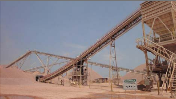
Photo 53: Crusher with safety signage and barriers.
