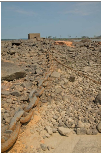
Photo 99: Anchor for the right-bank log boom.
