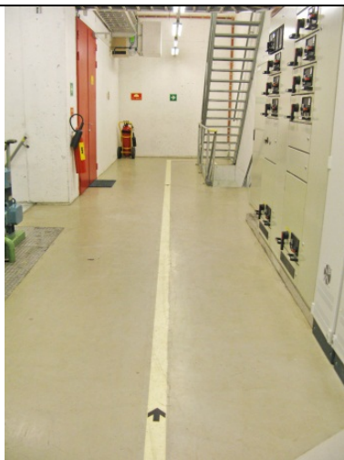
Photo 19: Clearly marked evacuation line on the floor in the power house
