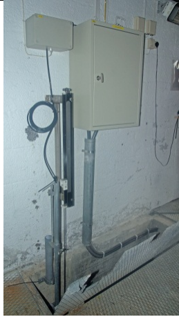
Photo 15: Automated measurement equipment for through-the-dam leakage
