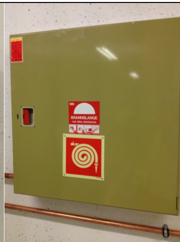
Photo 28: Fire-fighting hose, at the powerplant
