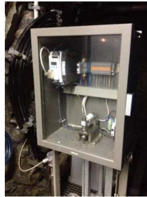
Photo 30: P-8 Dam movement monitoring instrumentation within Gepatsch dam
