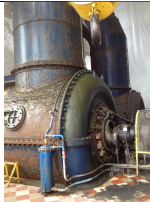
Photo 21: Original machinery at Les Vernes
