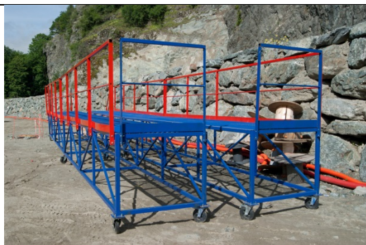
Photo 16: Loading platforms designed to reduce risk of unloading from truck, taken in response to a fatal incident
