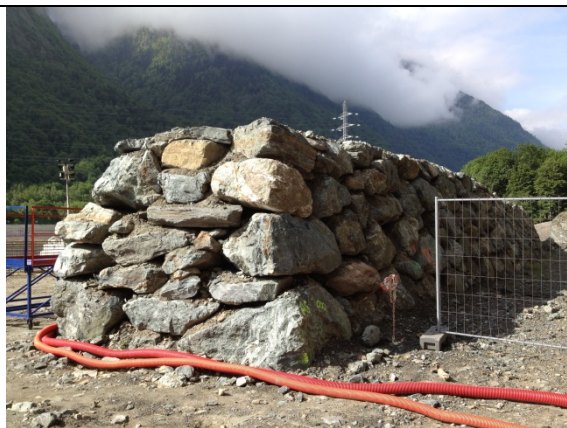
Photo 11: Stone wall constructed to prevent rockfalls from the cliffs from tumbling into the construction site
