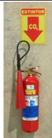
Photo 90: Fire extinguisher inside power house
