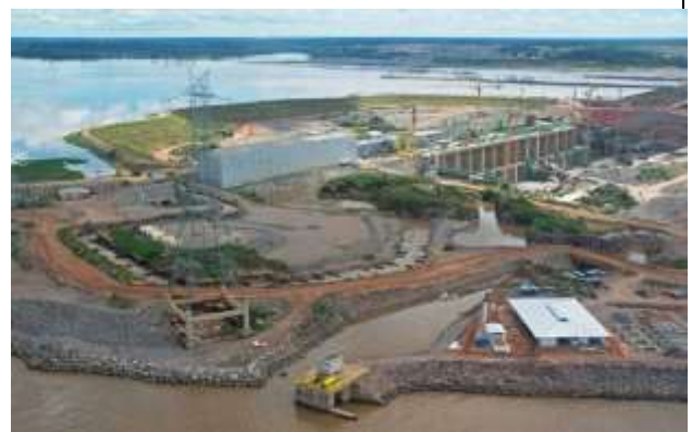
Photo 146: Aerial view of the right bank of construction site showing fish passage in foreground
