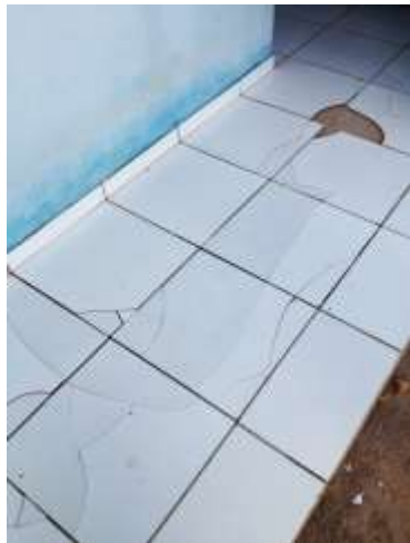
Photo 55: Parque dos Buritis, cracking tiling in several houses
