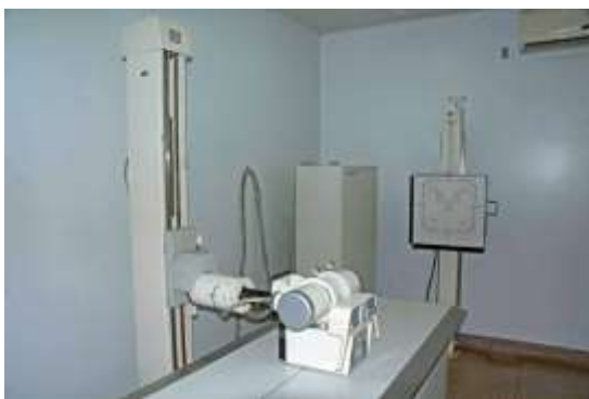
Photo 109: X-ray equipment in on-site hospital
