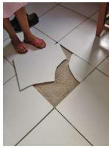
Photo 54: Parque dos Buritis, cracking tiling in several houses
