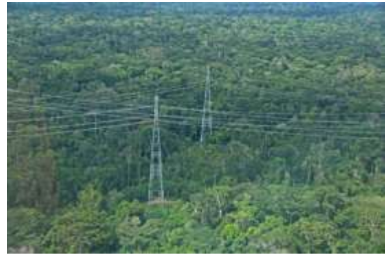
Photo 4: High-voltage transmission towers elevated to avoid impact on forest
