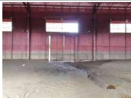
Photo 116: Historic warehouse EFMM after the floods
