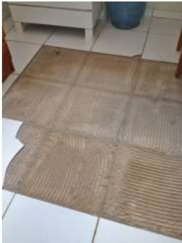
Photo 53: Parque dos Buritis, cracking tiling in several houses
