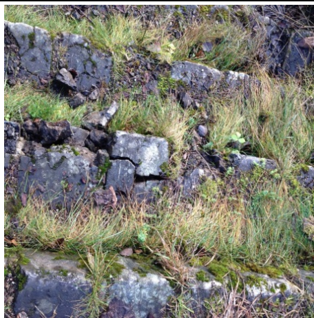
Photo 15: P-8, P-13, P-17 Deteriorating steps down to Semla II powerhouse present a tripping hazard for the public
