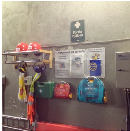
Photo 19: P-16 Safety equipment held within Semla III powerhouse.
