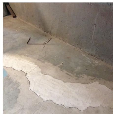
Photo 6: P-3, P-17 Indications of structural movement of Semla III powerhouse
