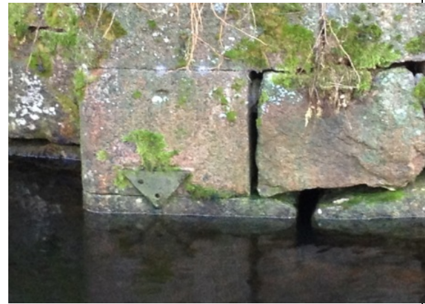
Photo 8: P-7, P-22 The arrow marks the permitted upper level of the reservoir
