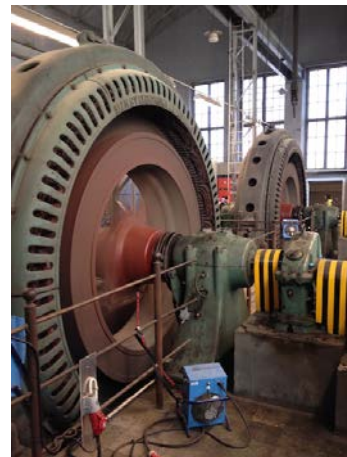
Photo 42: P-13, P-17 Historic generators in Semla III powerhouse
