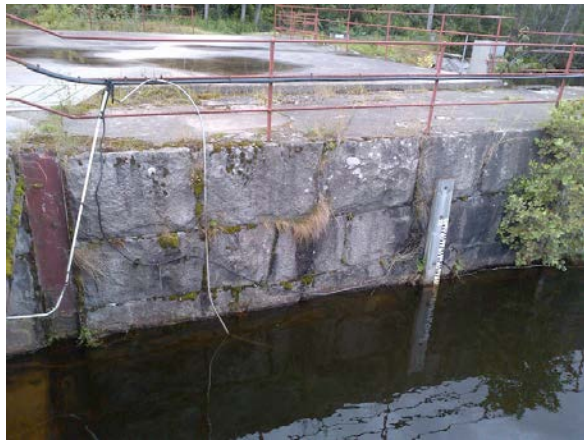
Photo 7: P-7, P-22 Water level gauges - wire and visual - on Semla Dam
