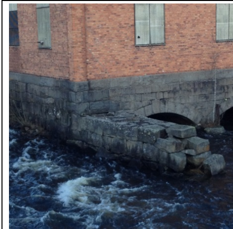
Photo 3: P-3, P-17 Poor condition of foundation of Semla III powerhouse
