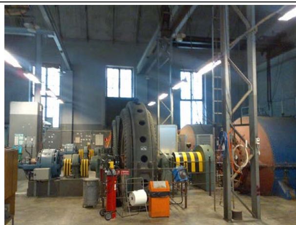
Photo 30: P-10, P-17 Semla III power house interior
