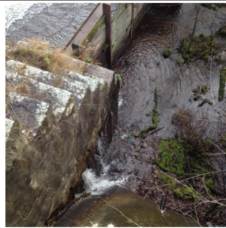
Photo 2: P-3 Leakage through the old part of the dam adjacent to Semla II powerhouse
