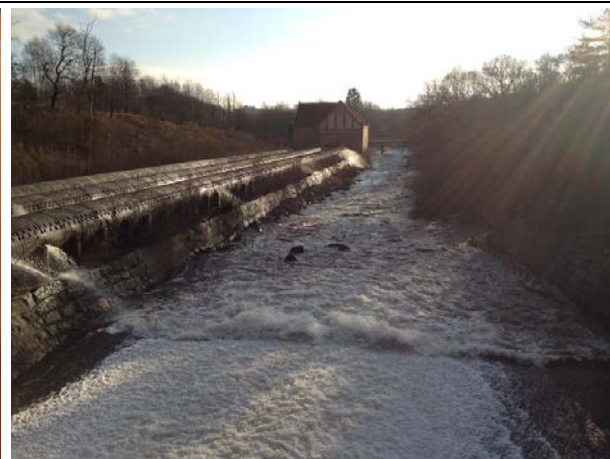
Photo 46: P-19, P-23 Flow during spill with penstocks and Semla III powerhouse
