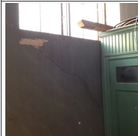
Photo 5: P-3, P-17 Indications of structural movement of Semla III powerhouse
