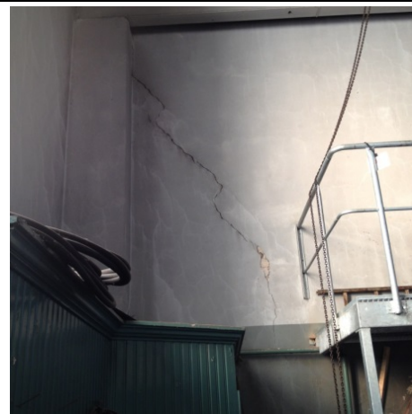
Photo 4: P-3, P-17 Indications of structural movement of Semla III powerhouse
