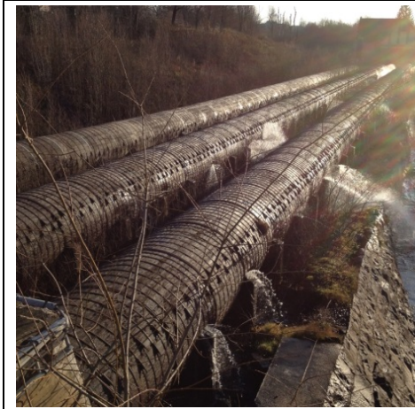
Photo 1: P-3 Existing penstocks in disrepair, indicating the need for rehabilitation
