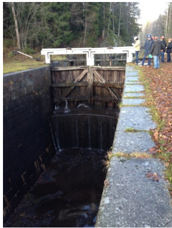
Photo 13: P-8, P-13 Canal lock showing potential falling hazard for the public
