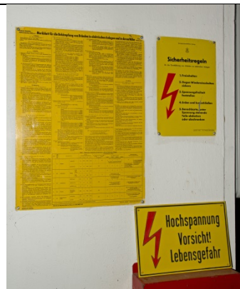
Photo 1v: Safety signage at Walchensee power plant, 28.02.2012
