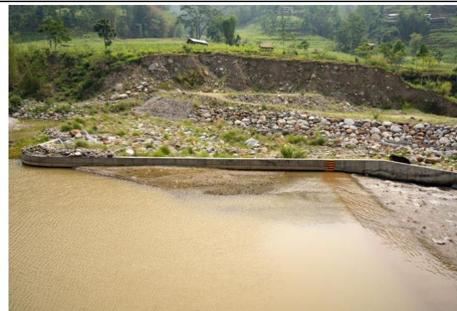
Photo 14: The bank erosion at the Mai Beni intake, caused by the outlet from the upstream project.
