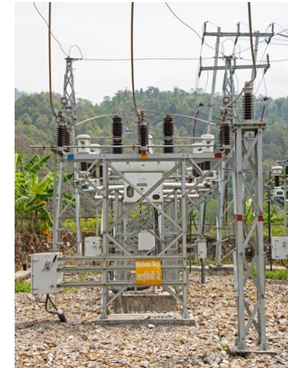
Photo 57: Mai Beni's incoming bay at the Godak substation.
