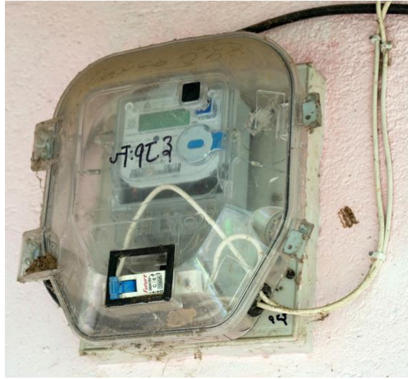
Photo 32: Electricity-connection box at the resettlement house.
