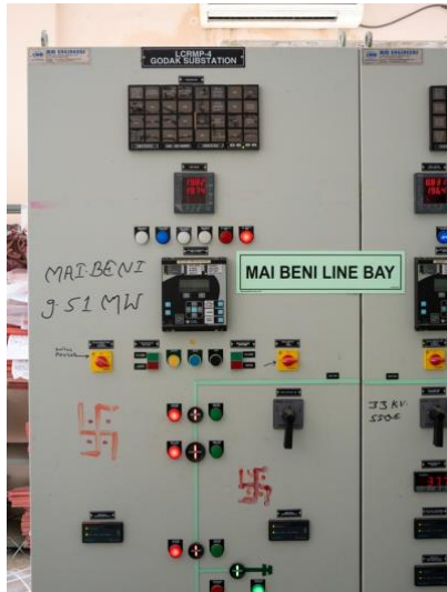
Photo 52: Mai Beni HPP's bay in the Godak substation control room.
