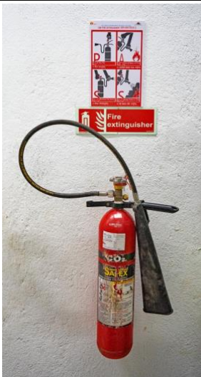
Photo 10: Fire extinguishers are found in several key locations around the plant.
