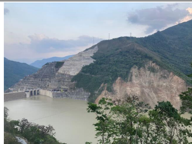
Photo 31: Dam and unstable areas on right bank
