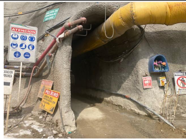
Photo 19: Safety signage and ventilation at drainage tunnel to stabilize slopes at 0+900
