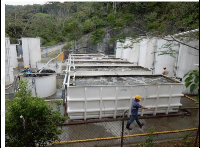
Photo 63: Wastewater treatment plant CCC camp
