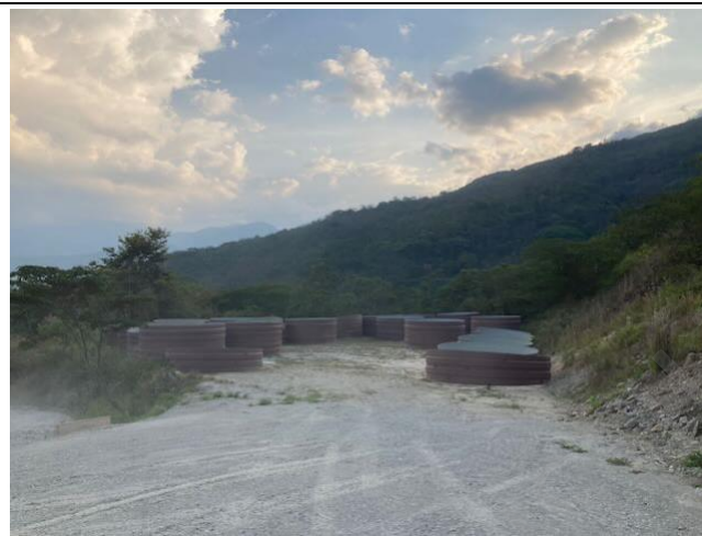
Photo 44: Storage of ferrules to repair intake sections damaged by the contingency, on left bank
