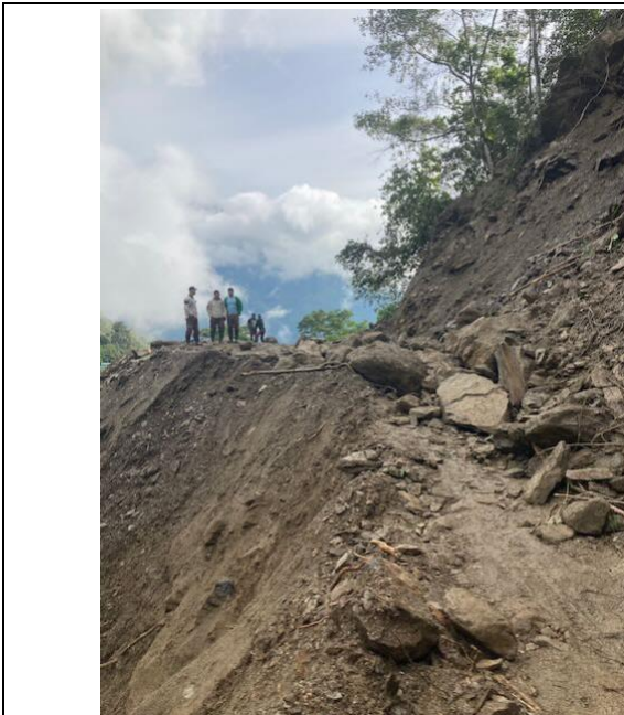
Photo 115: Typical landslide blockage, on road to Toledo rebuilt by EPM as community investment
