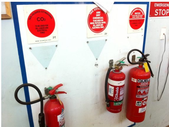
Photo 23. Fire extinguishers at Power Station
