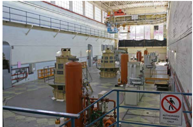
Photo 15: Inside Trevallyn Power Station
