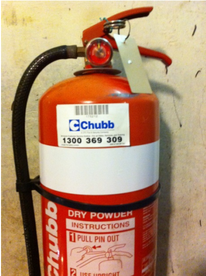
Photo 27. Fire-extinguisher, maintained in working order and with inspection labels, widespread at Power Station
